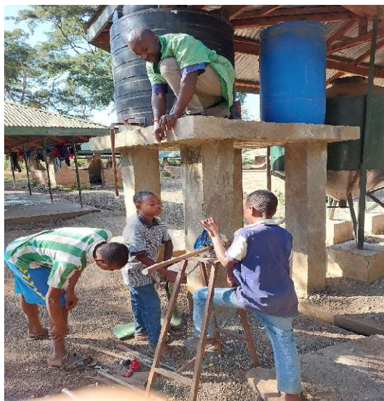
Plumbing activities near storage of water tanks
